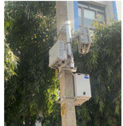
Demo Site with 2 Small Cell Installed
