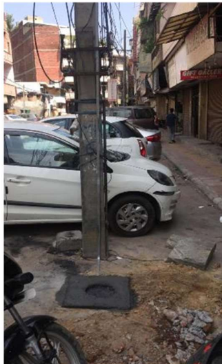
Maintenance free Earthing and Strip to poles with SC
